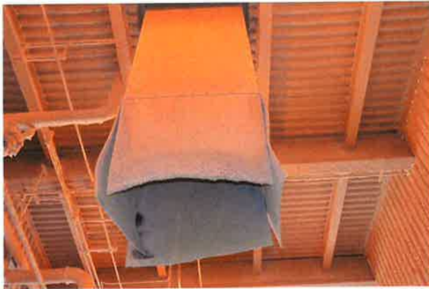
Figure 4.9 Truck Loading Spout for Pin & Paddle Mixer Discharge, extended for Fugitive Dust Control
