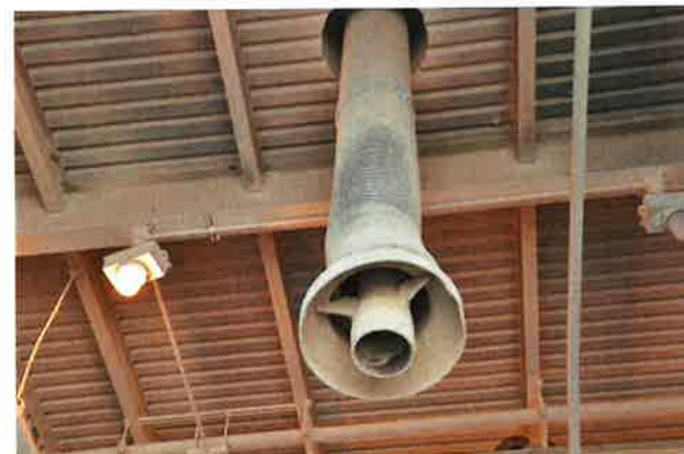
Figure 4.8 Typical Loading Spout in Truck Loading Bay at Ash Silos; Equipped with vacuum system and baghouse for Fugitive Dust Control
