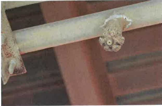
Figure 4.5 Spray Nozzle for Water Mist Curtain for Fugitive Dust Control at Ash Storage Silo Truck Loading Bay
