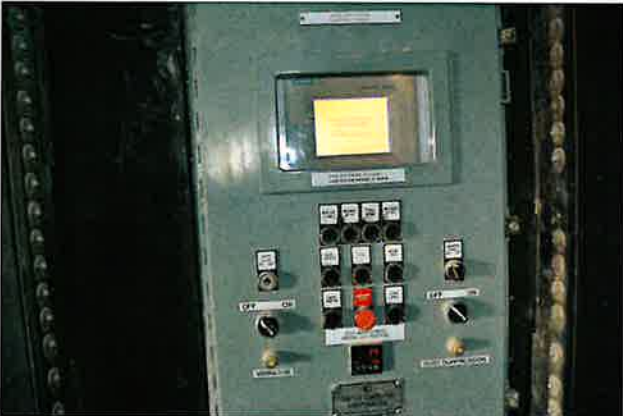
Figure 4.3 Control Panel for Pin & Paddle Mixer (Preparation of Conditioned CCR)
