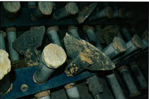
Figure 4.4 Interior of Pin & Paddle Mixer for Fugitive Dust Control (Preparation of Conditioned CCR)
