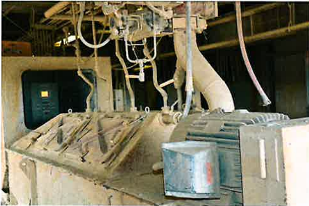
Figure 4.2 Pin & Paddle Mixer (Preparation of Conditioned CCR)
