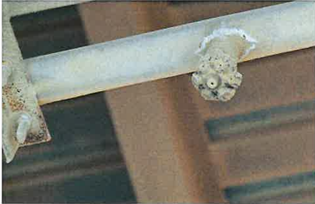
Figure 4.5 Spray Nozzle for Water Mist Curtain for Fugitive Dust Control at Ash Storage Silo Truck Loading Bay
