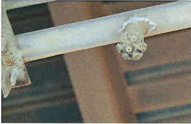
Figure 4.5 Spray Nozzle for Water Mist Curtain for Fugitive Dust Control at Ash Storage Silo Truck Loading Bay
