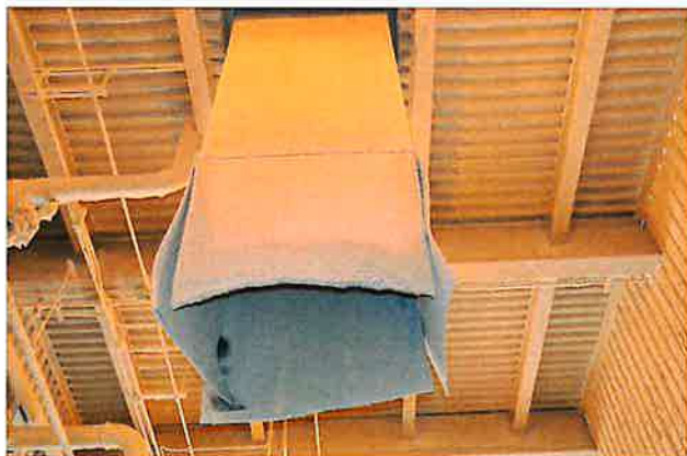
Figure 4.9 Truck Loading Spout for Pin & Paddle Mixer Discharge, extended for Fugitive Dust Control
