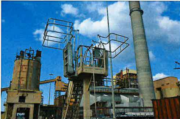
Figure 4.6 Truck Wash Station for Fugitive Dust Control
