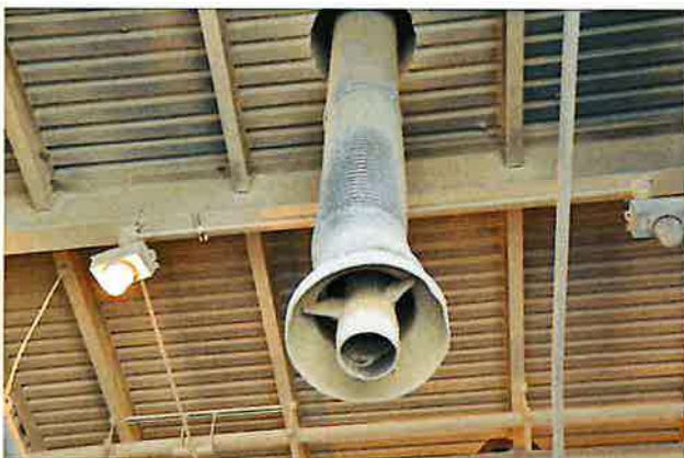
Figure 4.8 Typical Loading Spout in Truck Loading Bay at Ash Silos; Equipped with vacuum system and baghouse for Fugitive Dust Control
